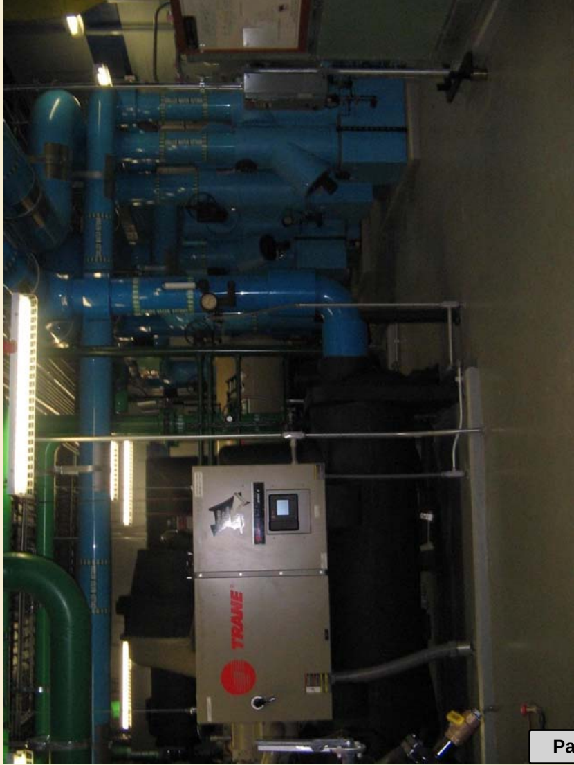
Deltona High Chiller Plant
