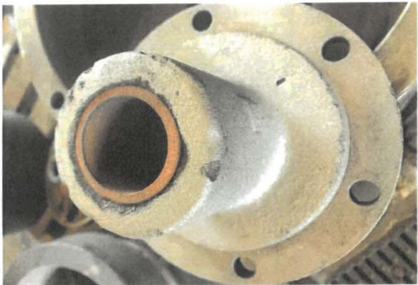
STUFFING BOX SHOWING SIGNS OF ERROSION
