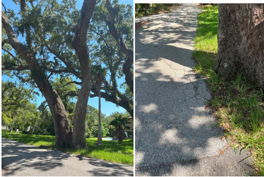
Tree #16 – Riverside Drive - Large root flare at road edge. May need air spade.
