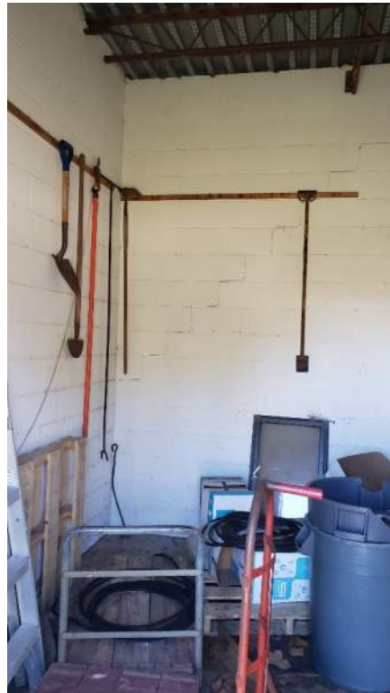
Stairstep Cracks at Masonry Wall at Custodial Storage
