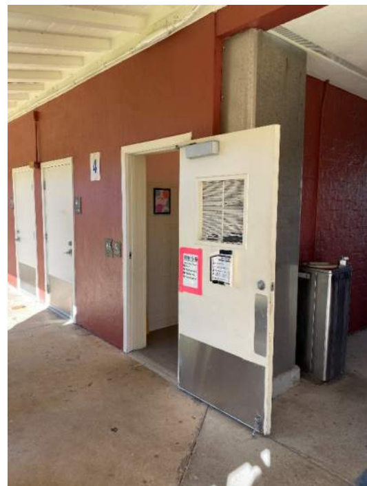
Restroom Door Swings Into Walkway
