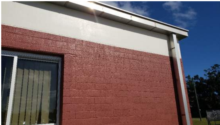
Cracks in Bricks at Window Exterior
