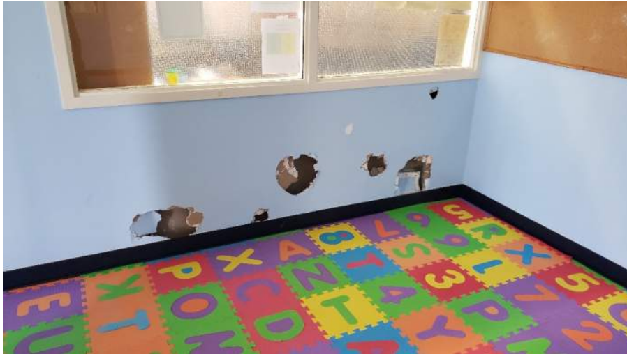
Dry Wall Damage in "Calming Room"
