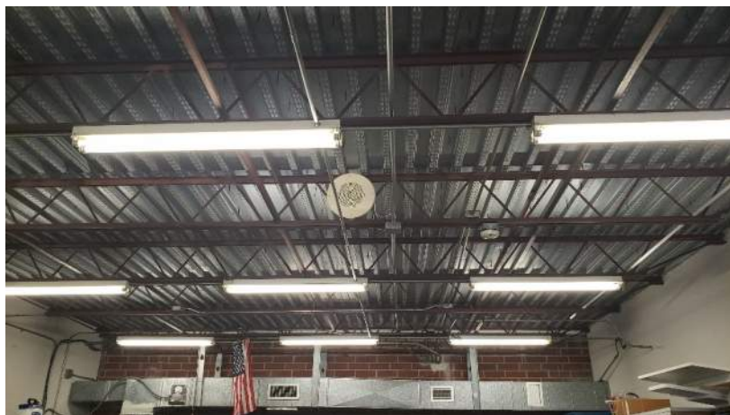
Ceiling and Ductwork in Custodial Storage
