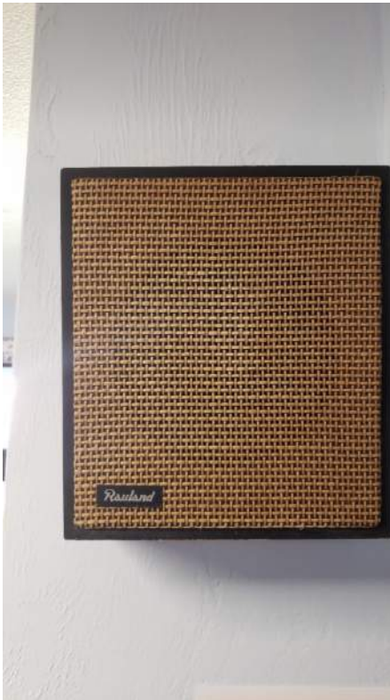
Outdated Intercom System
