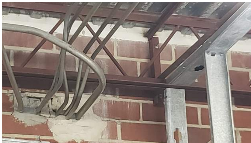
Wall Penetrations for Conduit in Rated Wall
