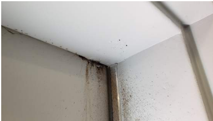
Moisture Intrusion at Exterior Wall
