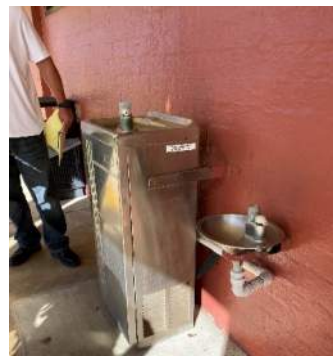
Non-compliant Drinking Fountains
