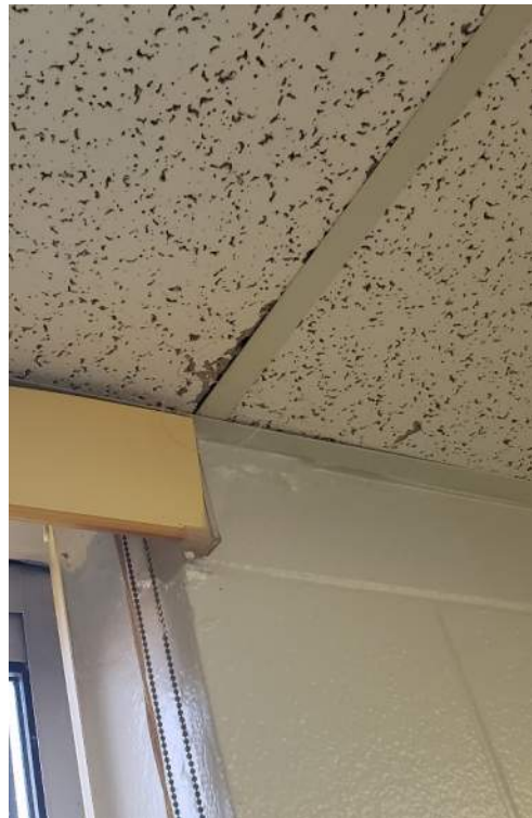
Moisture Intrusion at Windows Interior
