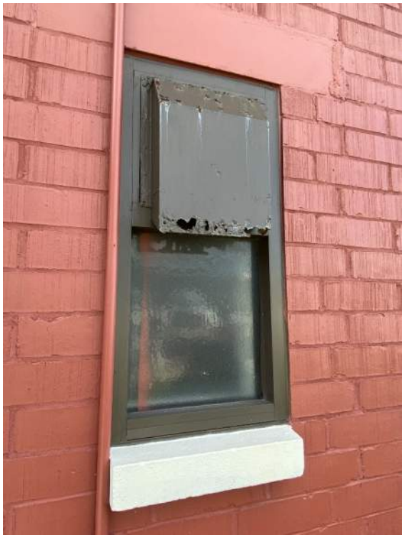
Exterior of Exhaust Fan
