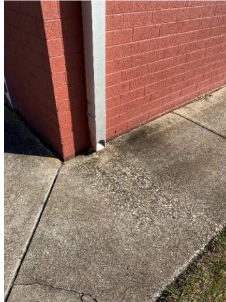
Downspouts Discharge to Cracked Pavement
