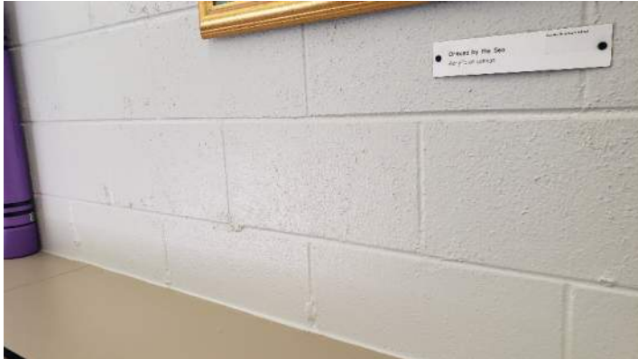
Moisture Intrusion at Floor Level
