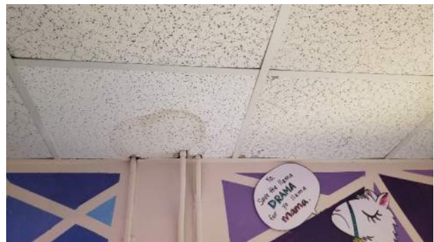
Water Damage on Ceiling Tile
