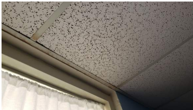
Rusting Ceiling Grid, Humidity Issues
